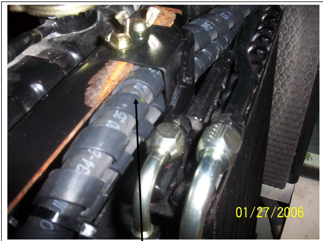
Hoses at condenser
